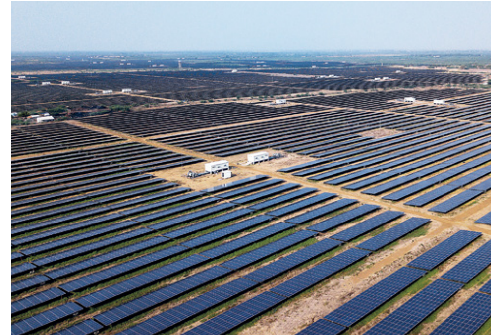
► Kamuthi solar power project, one of the world's largest, in Tamil Nadu
